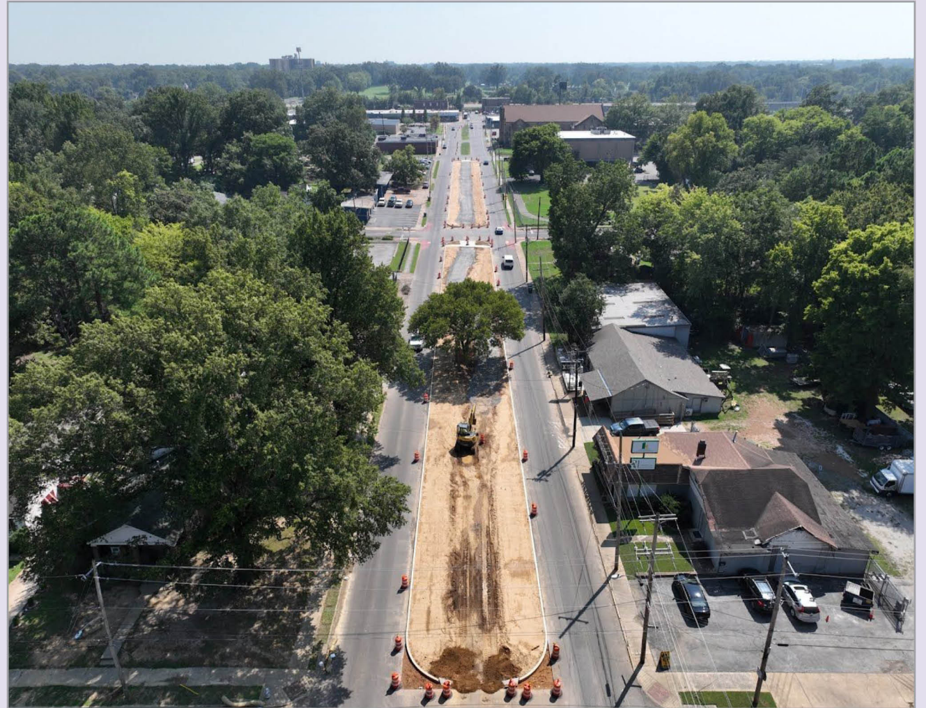
As part of the Highland Heights project, the Heights Line began construction in July 2023. Originally a vision spearheaded by the Heights CDC, the City is revitalizing a former trolley line into a multi-use trail that will be pedestrian and bike friendly. Construction will be complete early spring 2024. Photo by Malasri Engineering.
